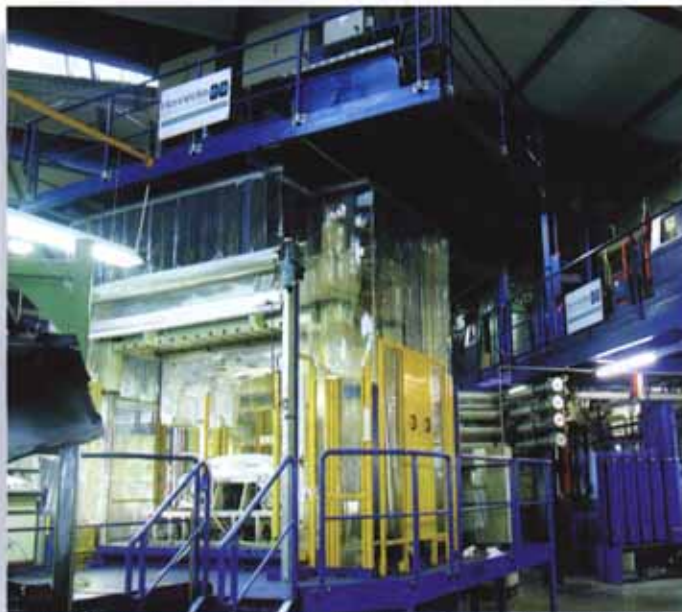
Rimdomat-FiberFlex production line in operation at KVG GmbH since October 2001.
